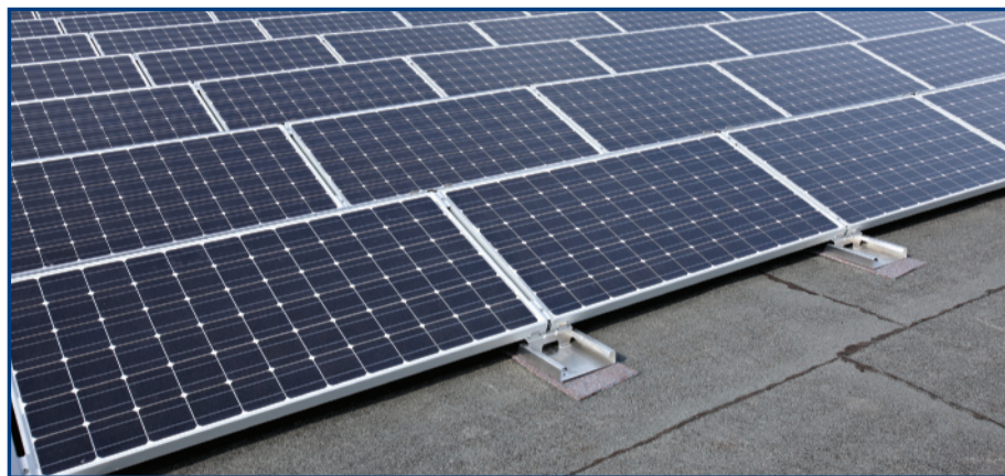
Figure 9.31: Solar photovoltaic panels at the 579 MW e Solar Star Power Plant in Los Angeles County, California. In contrast to most other large photovoltaic power stations, Solar Star uses single-axis tracking collectors rather than fixed collectors.
