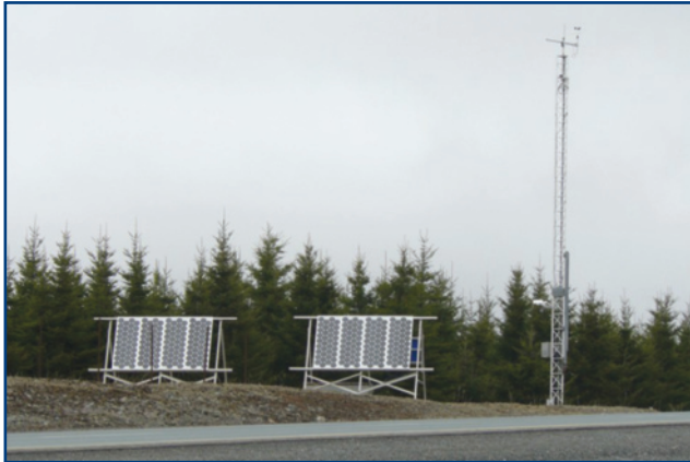
Figure 9.26: Photovoltaic array for providing power at a remote radio transmitter station.
