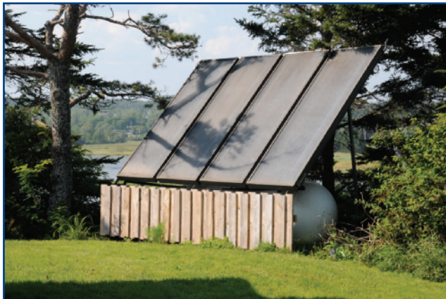
Figure 8.5: Flat plate solar collector installation.
